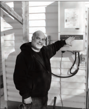
Craig Timmermans stands before the panel that interfaces between his generators and the grid.
